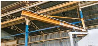
Demag 250kg Swing Crane #8
