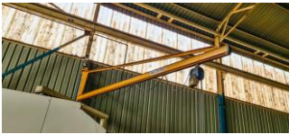
Demag 250kg Swing Crane #12
