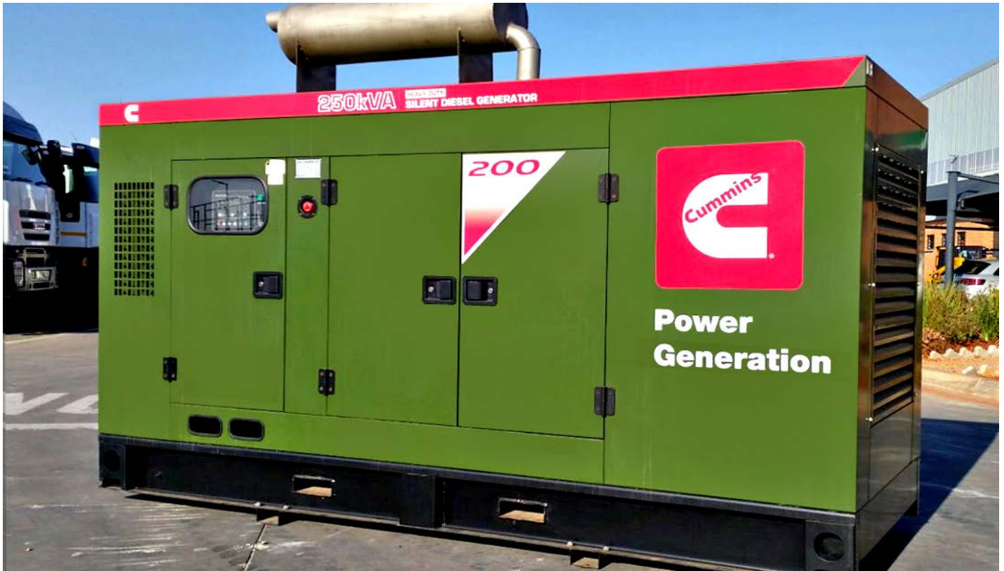
250, 160, 125, 75, 50, 38 & 15 kVA Diesel powered Silent Generators with ATS
