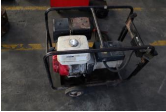
Turner Morris 6KVA Generator Faulty
