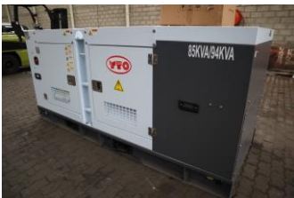
Cratos 94Kva YTO Silent Diesel Backup Generator with ATS Panel (Unused) Serial: *with Warrantee, Aluminium Diesel Tank & Galvanized Canopy* **Generator and Warranties- must be installed by WH Auctioneers approved technicians**
