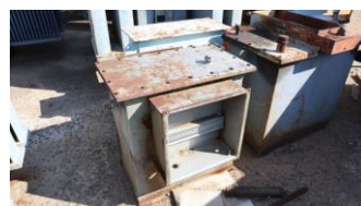
Lot of 5 Small Grey Transformers
