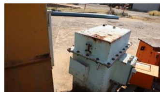
2 Small Grey Transformers
