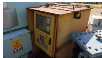
Battery Electric Charger Type LC (550Volt 31AMP)
