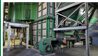
DB Thermal Rotary Dryer with Dutch Coal Furnace, Dual John Thompson Chain Stoker, 2 x FD Fan, Assorted Drum Drives, Control Panel and Assorted Ducting
