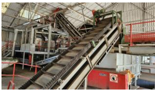
Buffer Bin with 3 x Auger Blades, De-Watering Conveyor and Pocket Conveyor
