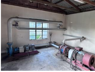
High Pressure Wash Feed with Pumps, 2 x 5,000L Filtration Tanks and Mobile Water Cannon
