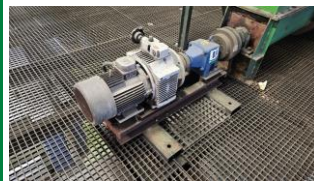
2010 BMG Variable Speed Drive
