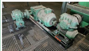
Lawrance Scott Variable Speed Drive
