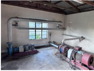
High Pressure Wash Feed with Pumps, 2 x 5,000L Filtration Tanks and Mobile Water Cannon
