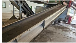
3 x Assorted Conveyor with Motor
