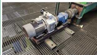
2010 BMG Variable Speed Drive
