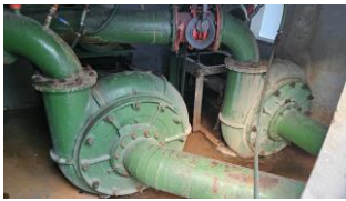
Water Pump Filtration System with 1.5m Roller Bed
