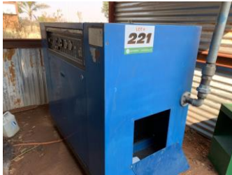
221 Stational Compressor with 2 Receiver Tanks
