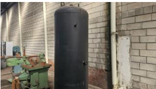
ILVA Air storage Tank
