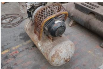
Compressor & Storage Tank
