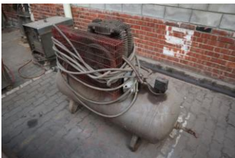
Balma Compressor and Air line Pipes
