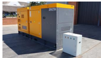
Cratos 275Kva SDEC Silent Diesel Generator with ATS Panel (Unused) Serial: 2216997 *with Warrantee, Aluminium Diesel Tank & Galvanized Canopy* **Generator and Warranties- must be installed by WH Auctioneers approved technicians**
