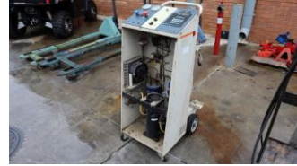
Smartcharge Aircon Filling Station - Damaged
