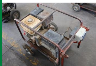
Malvon 6KVA Generator Engine Low Compression
