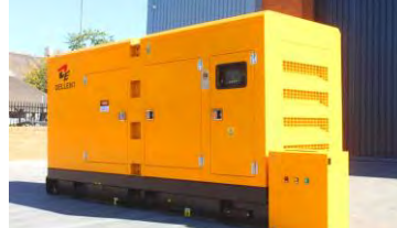
Dellent 250kva Silent Diesel Generator- Unused With ATS, Built in Diesel Tank, 3 Phase and Silent Enclosure
