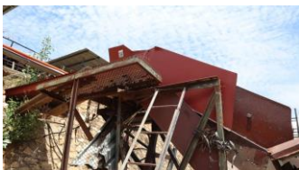
Conveyor to Fuel Bin SLM_WM_WS_15
