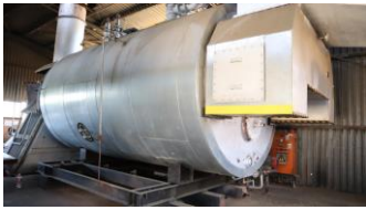
*STC*1975 Standardkessel Boiler with Control Unit
