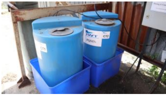
Chemical System for Both Boilers IWT Control Panel(Chemical System)
